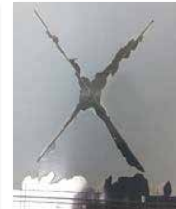
Aluminum panel made from alloy Y shows poor adhesion & significant delamination of paint from the surface
